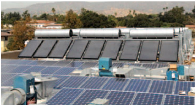
Figure 6 Solar PV and thermal collectors on the same roof [127]
